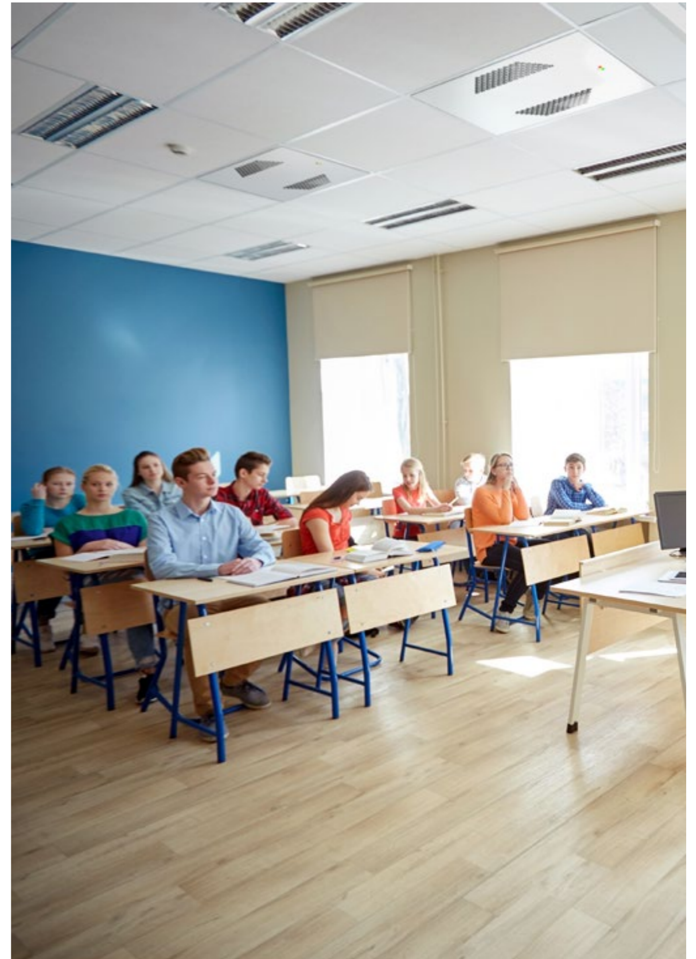
Application of UV-C Sterilon Square PP luminaires in classrooms
