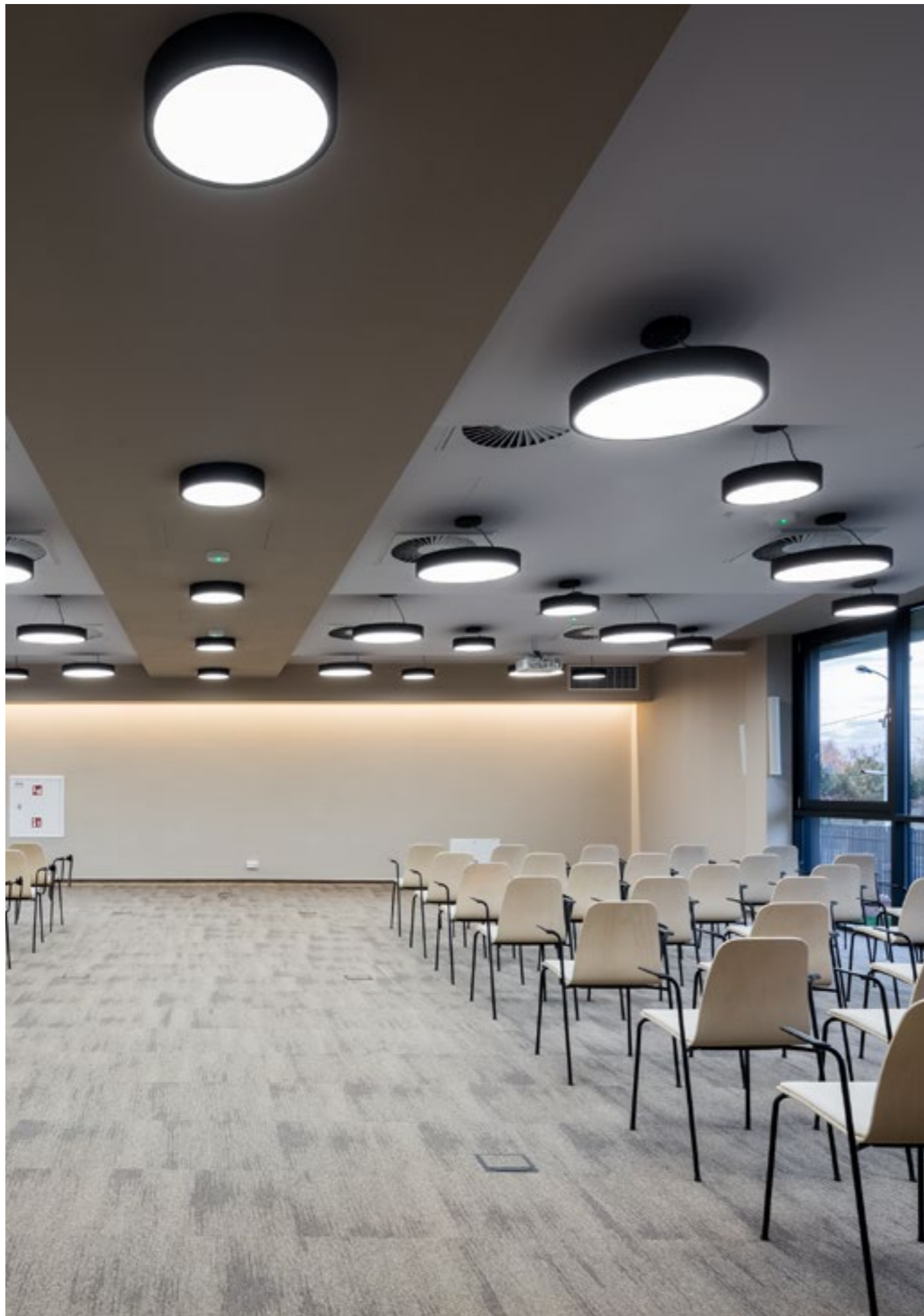
The application of the Coria LED system in the conference room at the African Missions Centre in Borzęcin Duży
