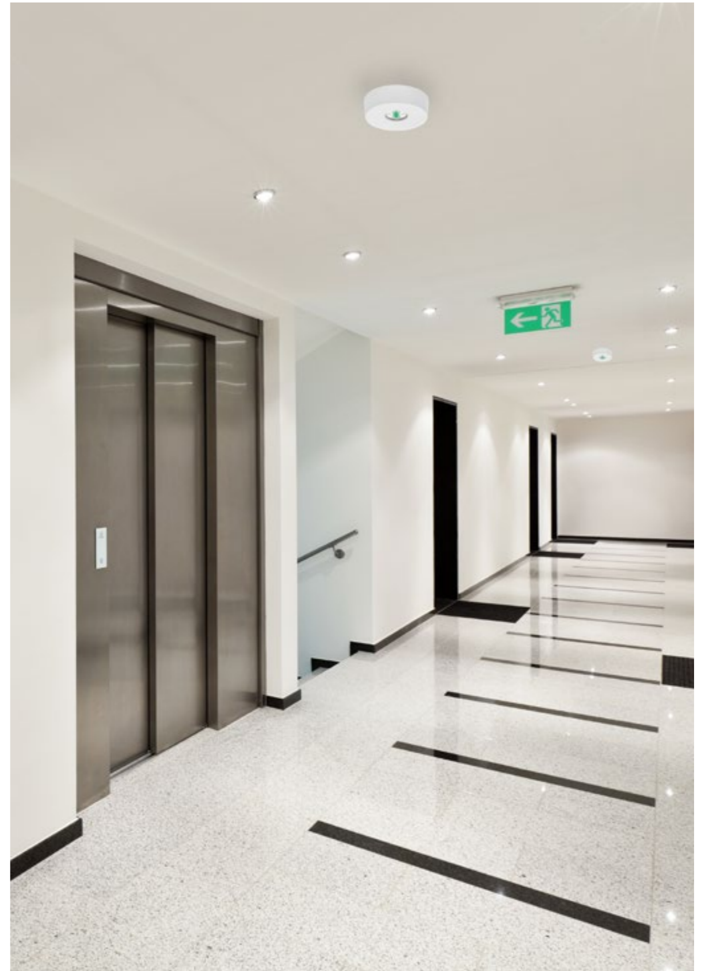
Application of the DOT CS LED luminaire in a corridor of an apartment building.
